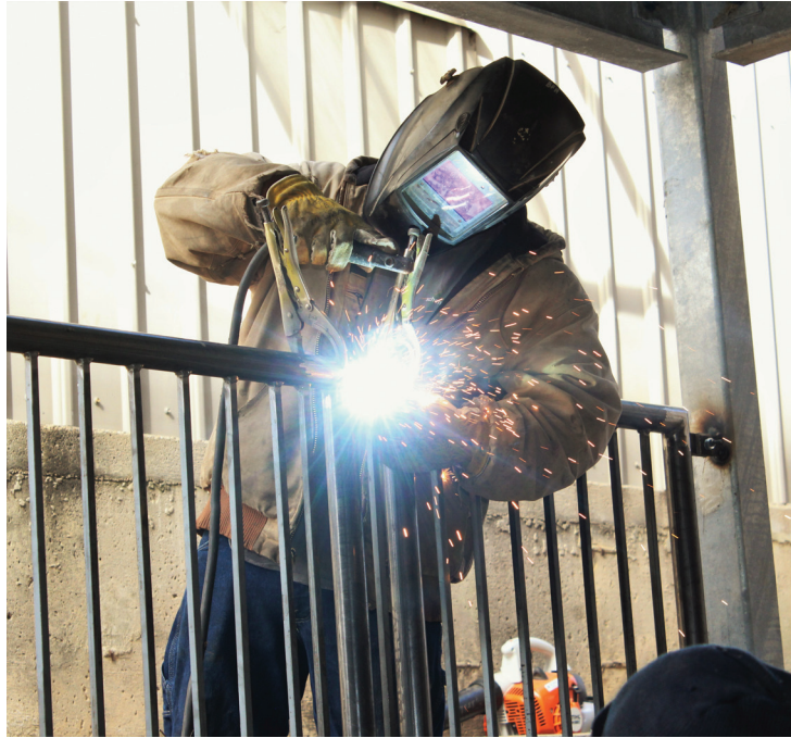
Brett Hutton welds a bracket while installing the new steel railings at the Auditorium. Photo by Dennis Crispin
